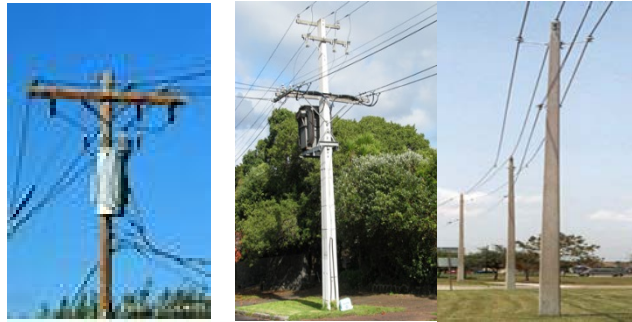
Existing Pole Hardened Pole Hardened Pole
